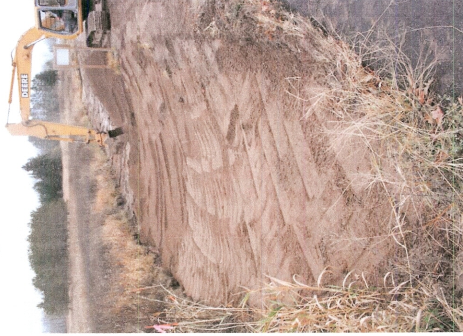
Photograph 4. Placement of clean gravel fill followed collection of confirmation sampling of sub-base. Placement of gravel fill was placed from west to east beginning November 6, 2008. Photo taken facing east.
