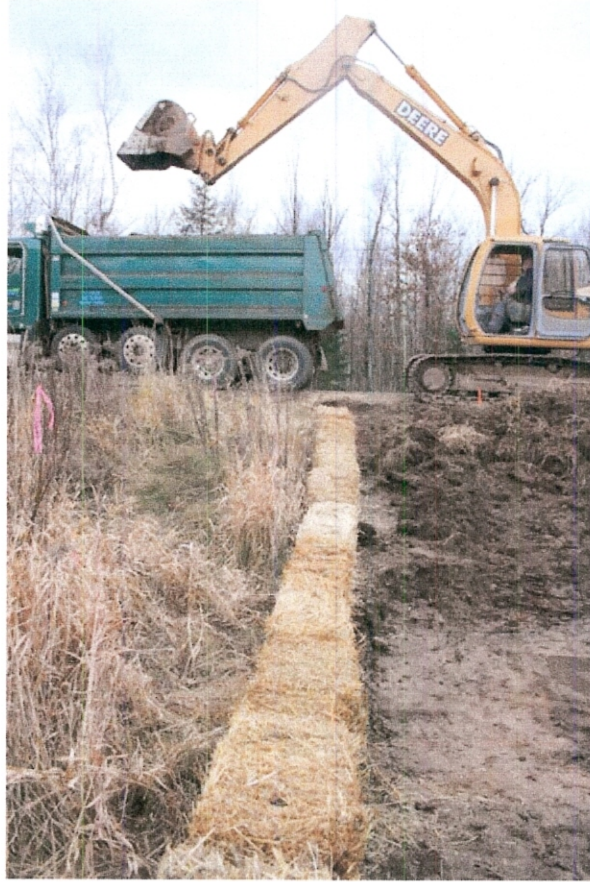
Photograph 1. On November 5, 2008 work began with the installation of a strawbale fence prior to excavation of surficial soils from the Copper Park Lane north ditch. Photo taken facing south.
