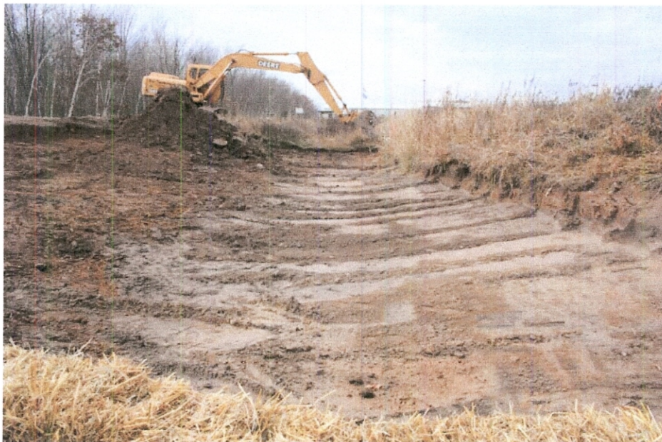
Photograph 2. The Copper Park Lane ditch surficial soils were excavated from east to west beginning on November 5, 2008. Photo taken facing west.
