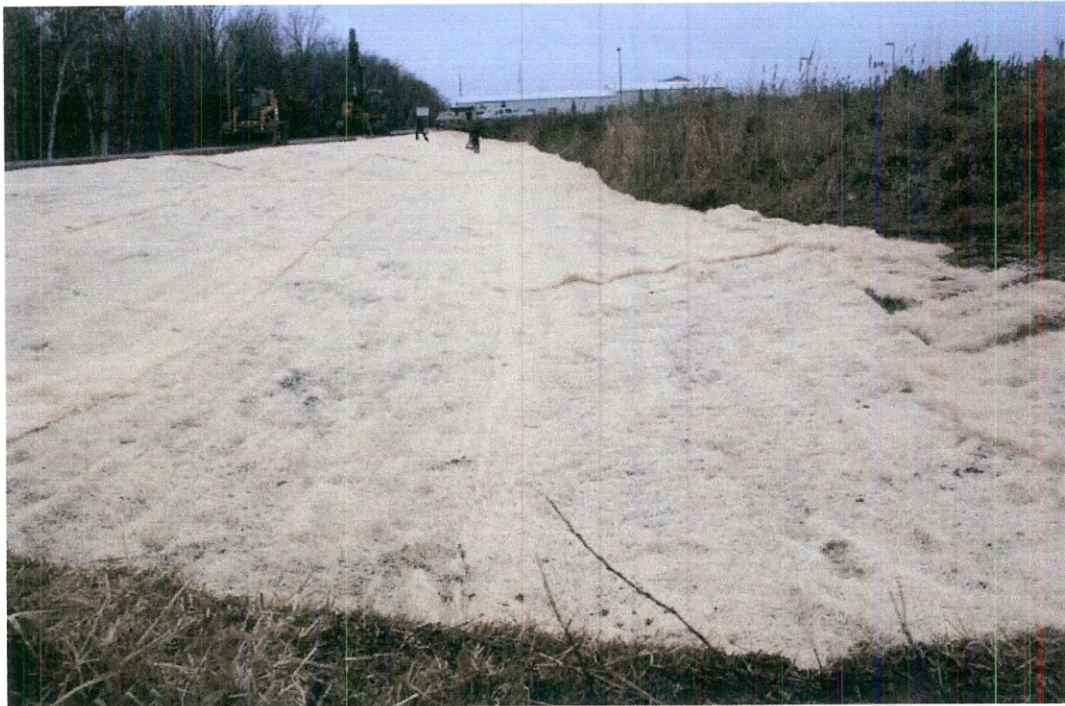
Photograph 7. Netfree erosion control blanket was installed across the entire disturbance area and secured with biodegradable stakes by end of day November 7, 2008. Photo taken facing west.
