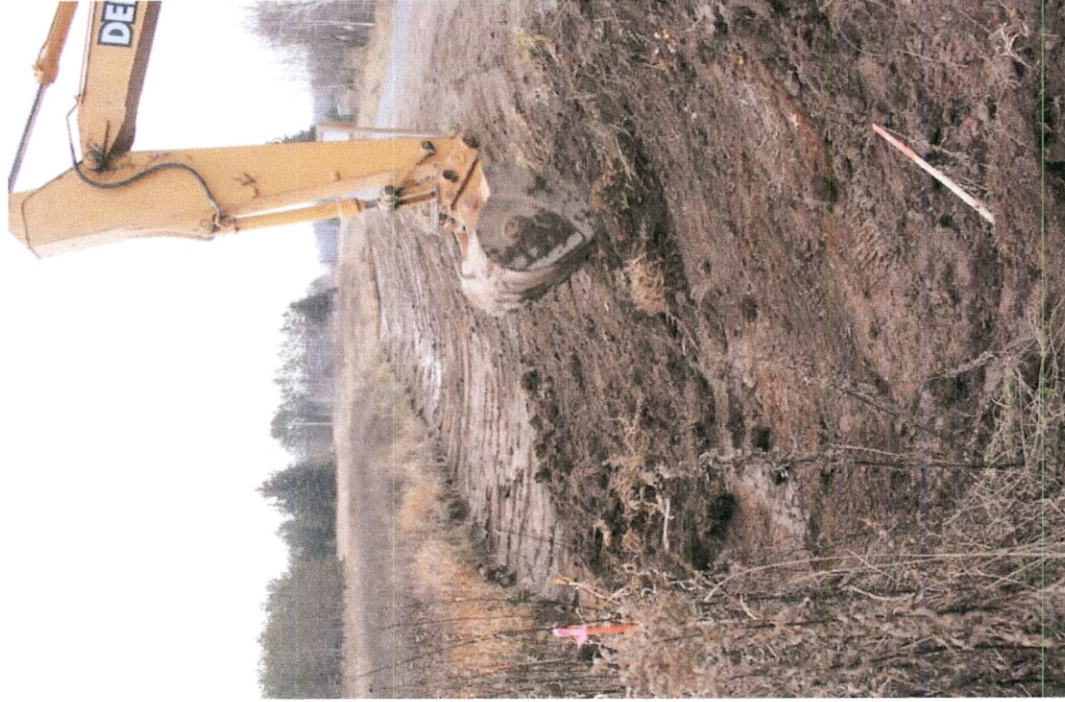
Photograph 3. Excavation of surficial soils was complete on November 6, 2008 ending at the western most end of the Copper Park Lane north ditch. Photo taken facing east.
