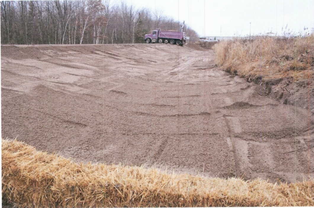
Photograph 5. Placement of gravel fill was completed on November 7, 2008 and placement of topsoil was immediately begun. Photo taken facing west.
